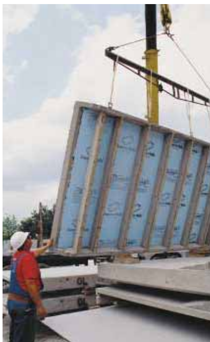
The insulated precast wall panels are lifted into place with a crane, producing a fast foundation wall that speeds construction. Its monolithic design also eliminates more opportunities for water seepage.
