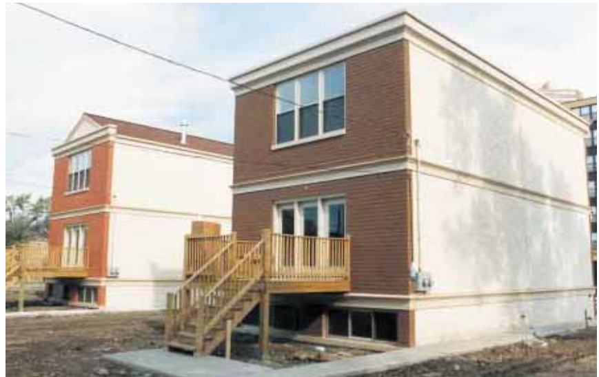
The panels feature brick-like textures on front and back, while the sides are painted and textured to fit with the typical style of these homes in the neighborhood.
