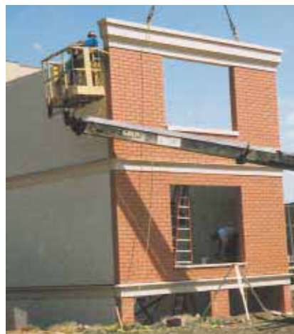
The precast panels produced by Prestress Engineering Corp. are trucked to the site as one unit. The 18 pieces required to assemble them can be erected in one day.
