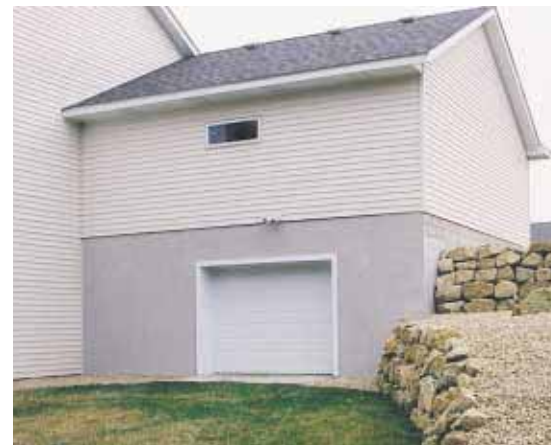
(Above) A room can be added under a new home by spanning the space with precast concrete hollowcore slabs.
